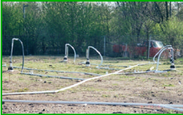
Figure 5. Soil Vapor Extraction (SVE) System.
