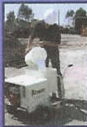
ORC slurry is poured into the hopper of a Slurry Injection Pump.
