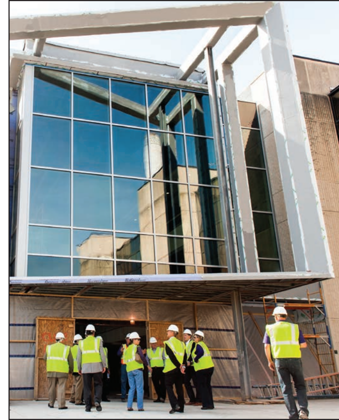
Members of the college's advisory council and college staff look at the progress of Phase IV.
