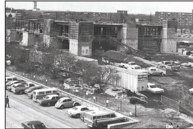
Construction nears completion on Durland Hall, soon to be the home of the K-State departments of chemical and industrial engineering.
