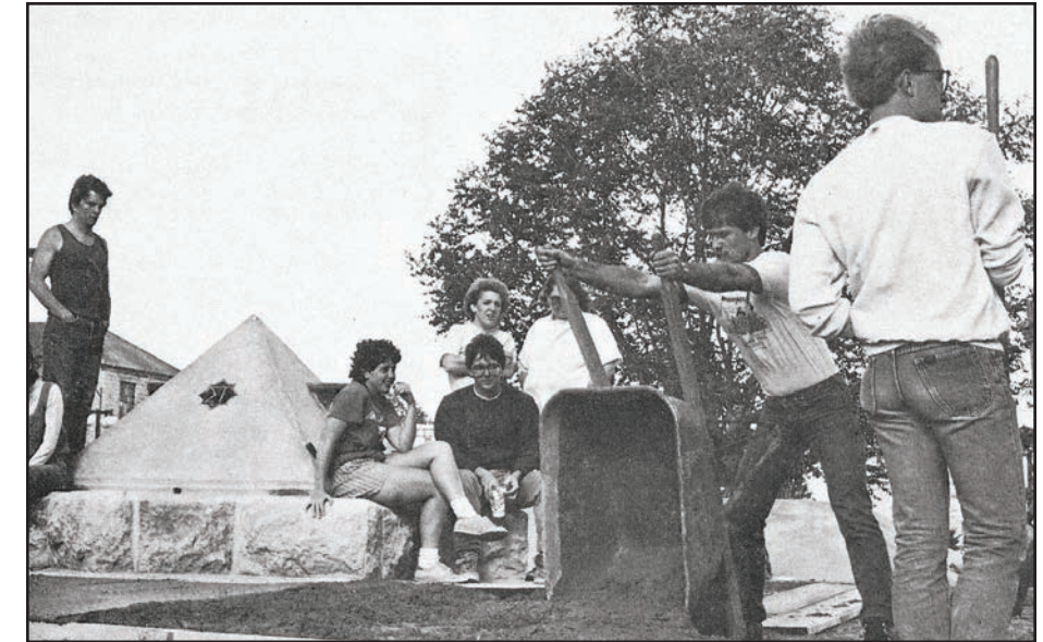
The old Sigma Tau pyramid got a new resting place in March when it was moved from a site near Seaton Hall to one next to Durland Hall. Taking on the relocation project were members of the student chapter of Associated General Contractors.
