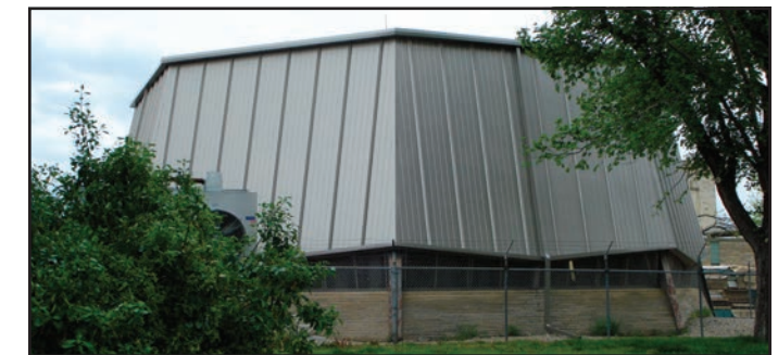
An outdoor view of the newly replaced reactor walls shows an improved system of panels rated for 90 mph winds, with replacement following the June 2008 tornado.
