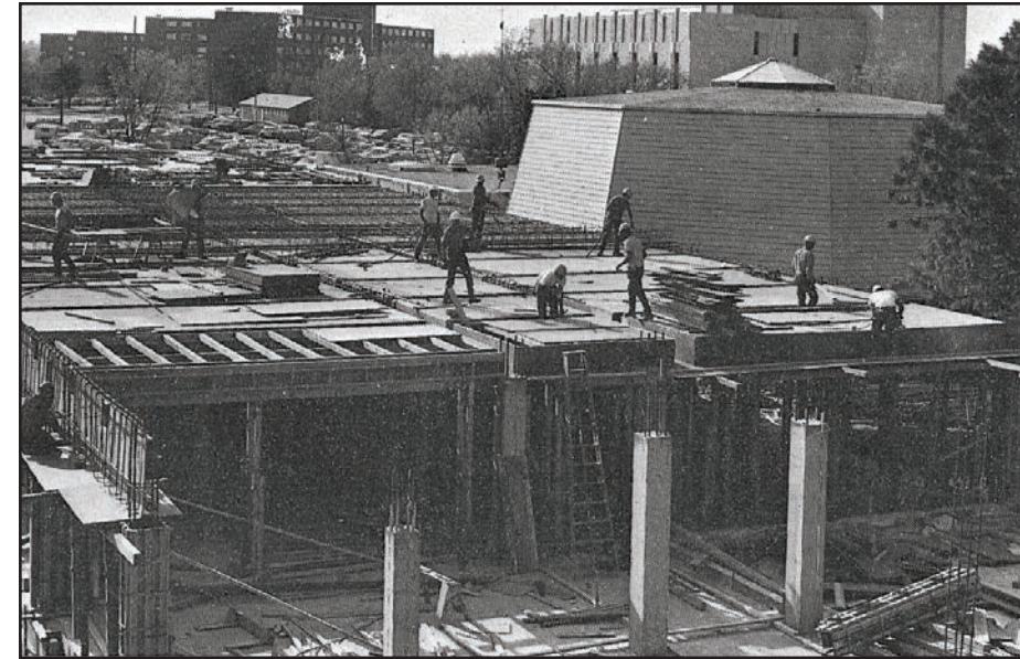
Construction on the Ward Hall addition, valued at nearly $1 million, continues "right on schedule," slated for occupancy next fall.
