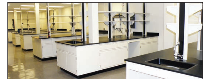
Newly renovated engineering labs in the basement of Seaton Hall were occupied for use in the 2013 fall semester.
