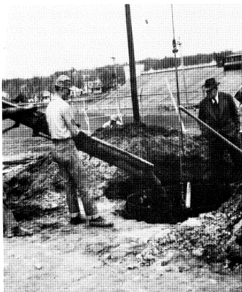
Seaton supervised the construction of nearly two dozen buildings on campus during his long career. An authority on concrete, here he watches the pouring of a concrete pedestal on the field house in 1949. (Courtesy of the Seaton family.)
