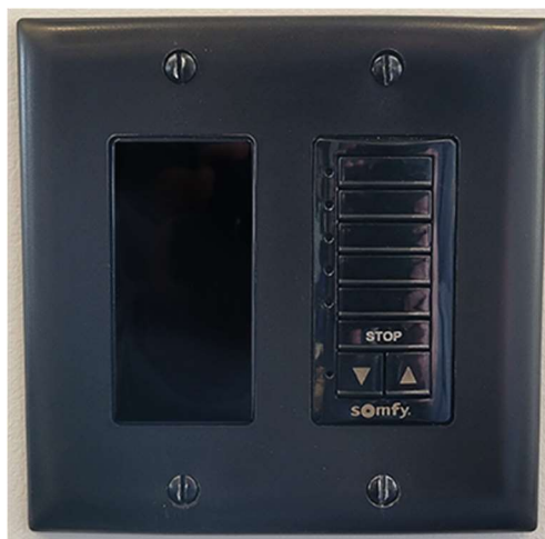
Window Shade controls
