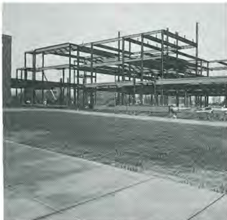
Durland Hall, Phase II, a three-story structure, will be connected to the north end of Durland, Phase I by a lobby.
