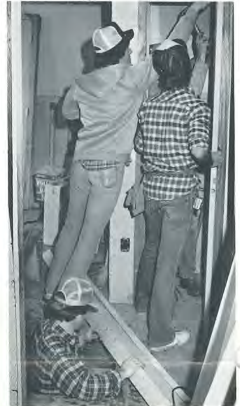
Construction science students work on doorframe of three-room home addition they are completing as a project for their chapter of Associated General Contractors.
